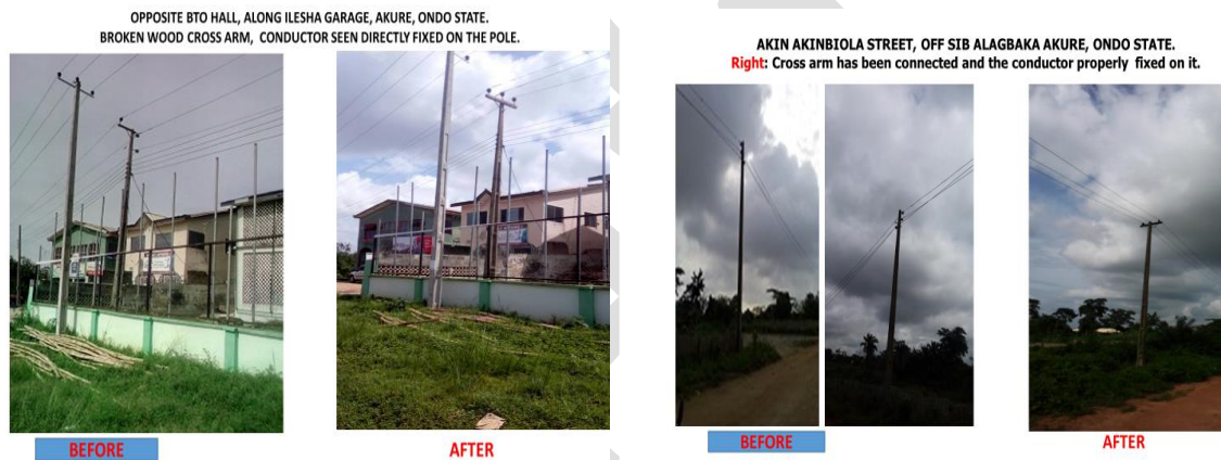
Figure 9: Samples of BEDC In-House Network Defects Observations/Resolution
